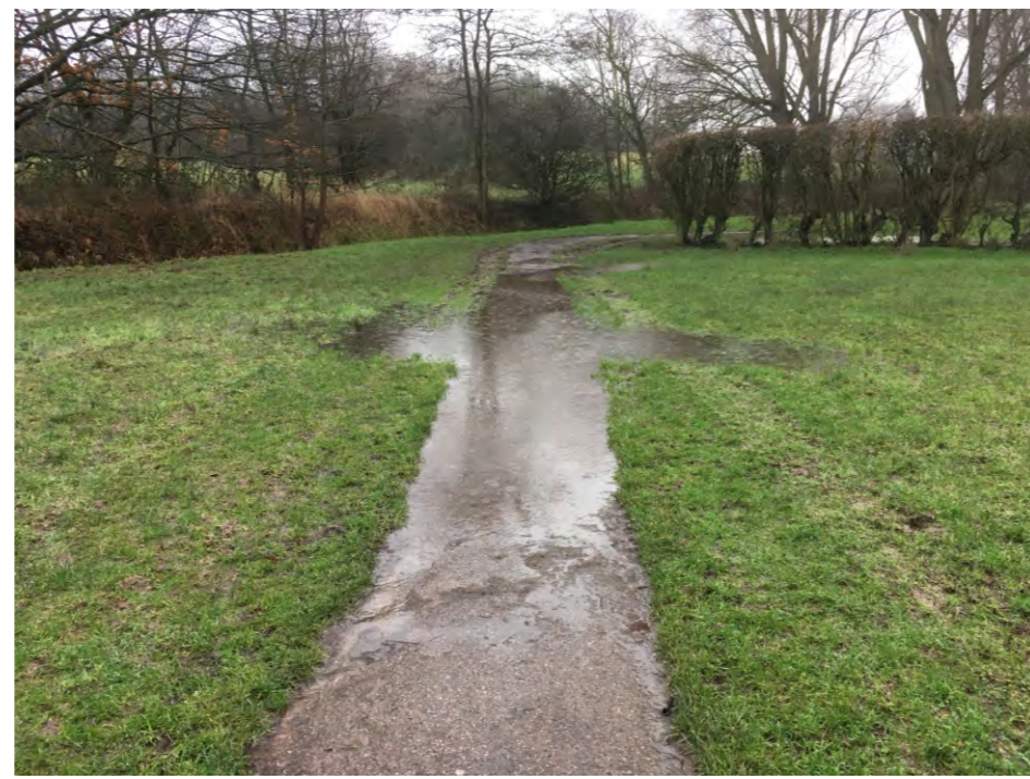
2. Footpath drainage problems.
