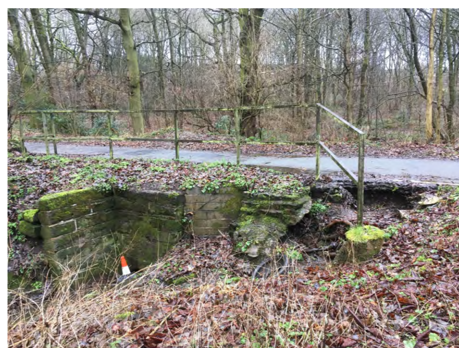
19. Existing brook headwall in poor condition.
